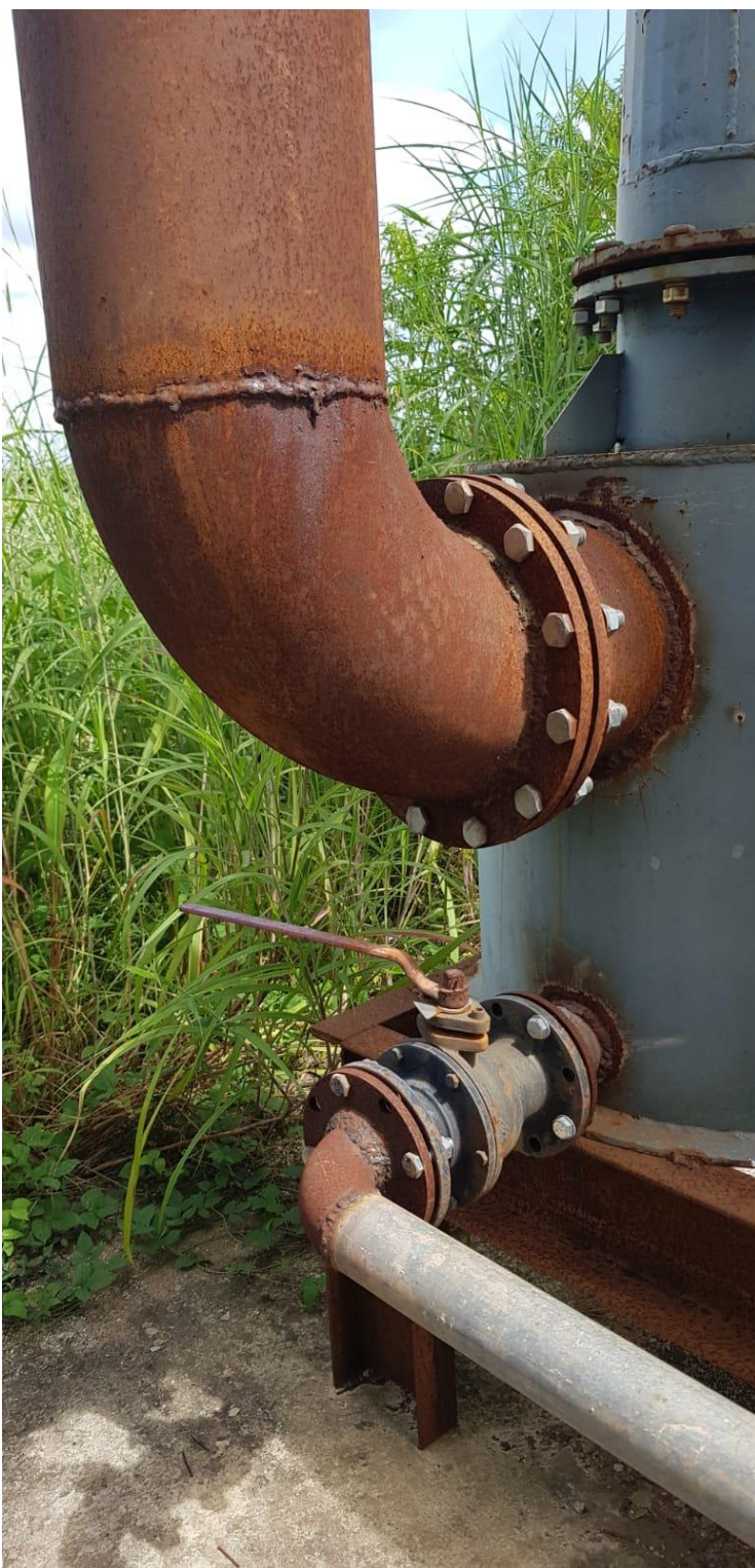
Extent of corrosion and poor welding on some of the pipework
