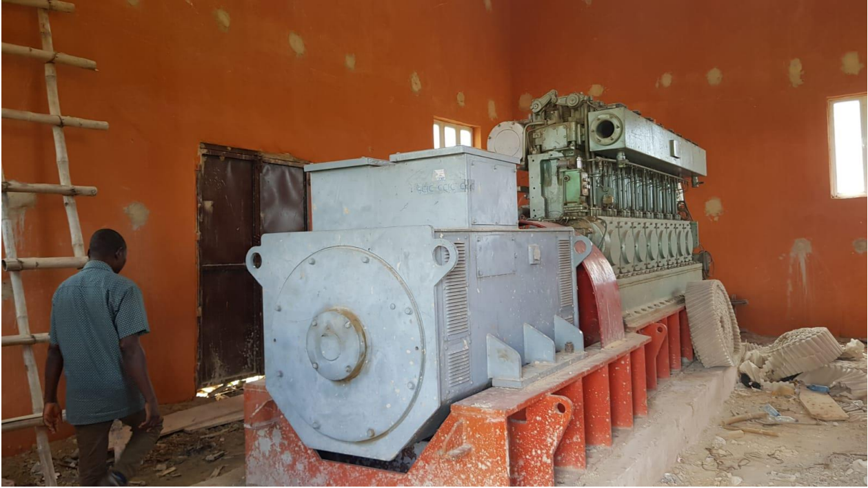
Condition of storage of 0.5 WM engine and generator
