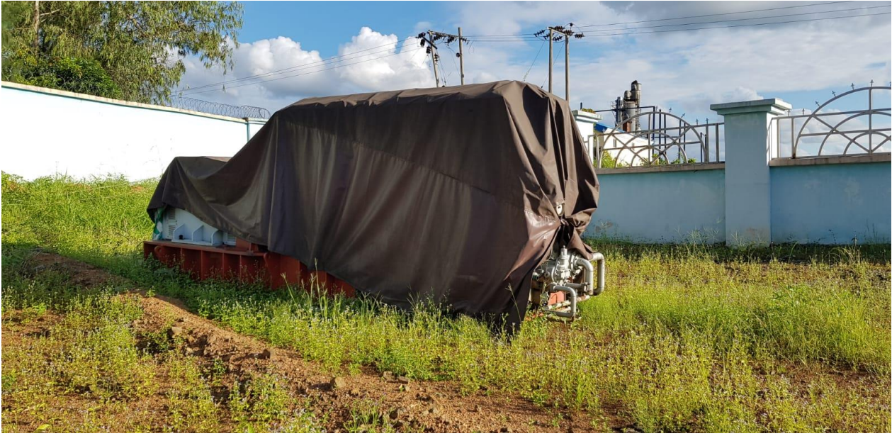
Condition of storage of 1 MW generator
