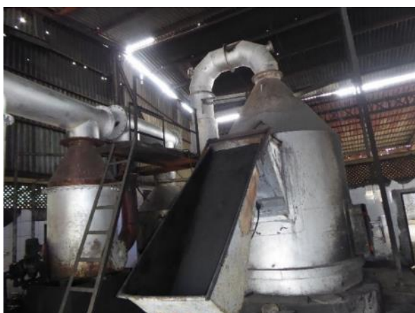
The incinerator (right) and the start of the APC left
