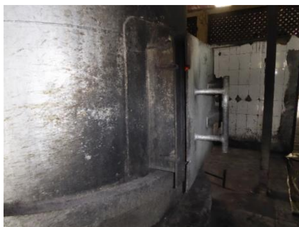
Waste is fed into the combustion chamber through this door
