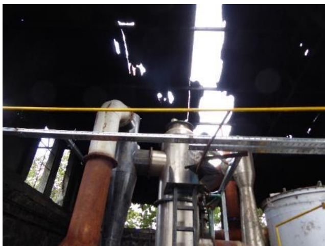
The air pollution control system under a leaking roof
