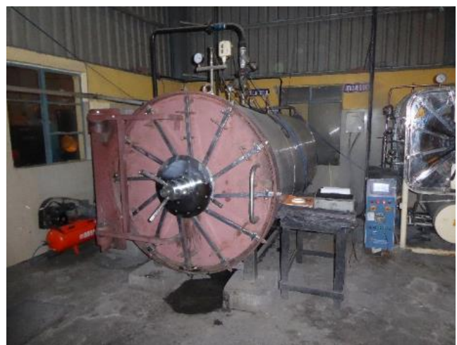
Two of the facility's autoclave units.
