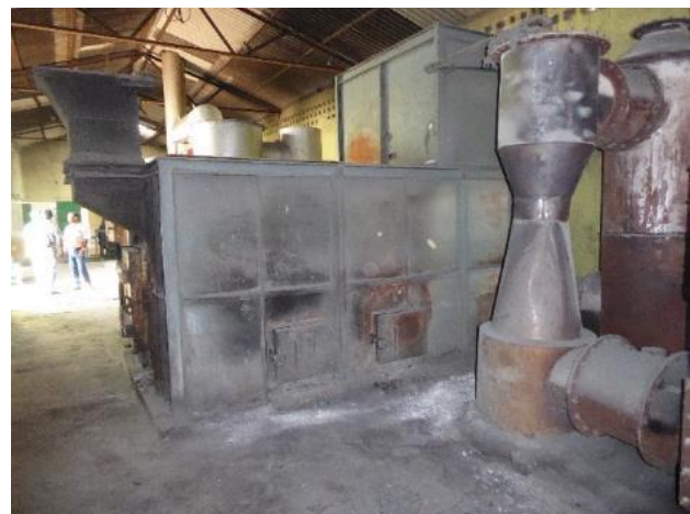
One of the facility's two incinerators, the waste is fed through the access door in the centre of the picture.
