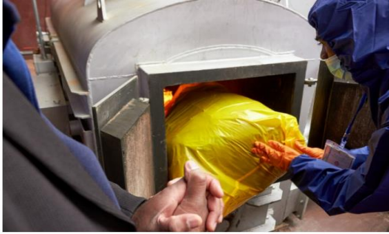
Country: Madagascar Company: Chuwa Industrial Co., Ltd. Hospital staff using the incinerator
