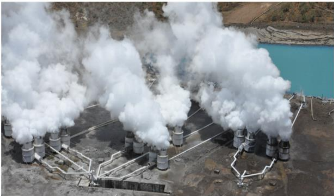
Figure 3: Menengai well MW-1A under discharge test using seven twin separators to handle the large total mass produced. The well produces steam equivalent to 30 MW electric when on full discharge
