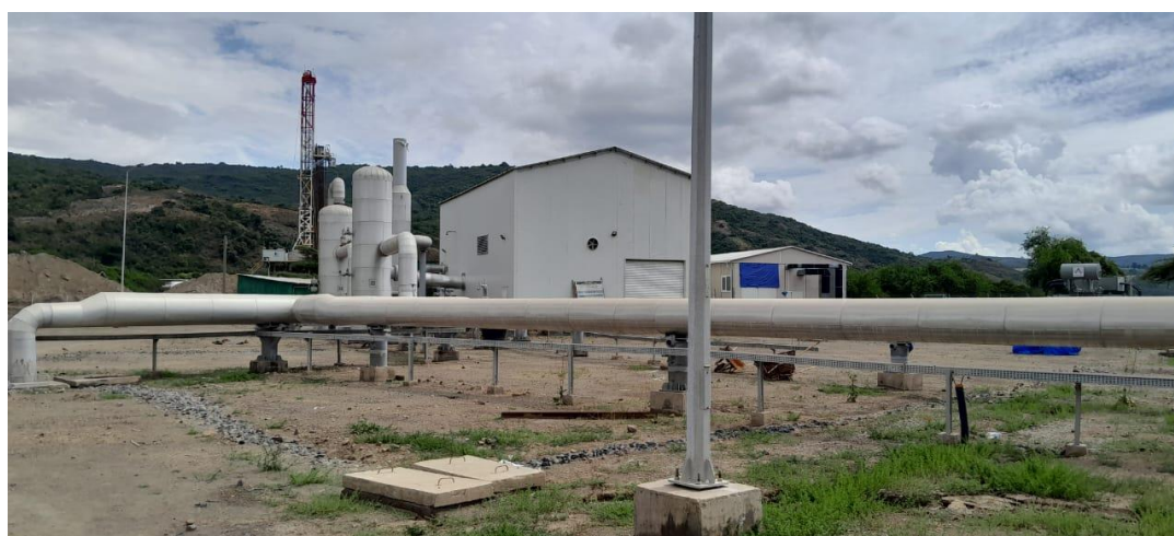
Figure 8: Aluto 5MW plant to be commissioned in 2023
