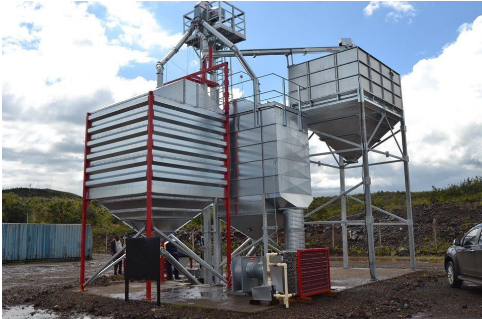
Figure 25: Grain dryer utilizing geothermal steam at Menengai (Source: GDC)
