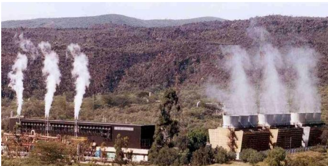
Figure 6: A view of Olkaria 1 power plant located in the Olkaria East production field
