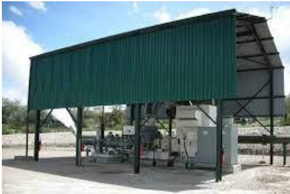
Figure 12: Photo of Oserian Back Pressure, 1.8 MW Gross power plant
