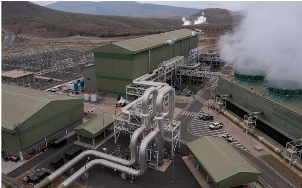
Figure 10: Photo of Olkaria V, 173.2 MW Power Plant commissioned in 2019
