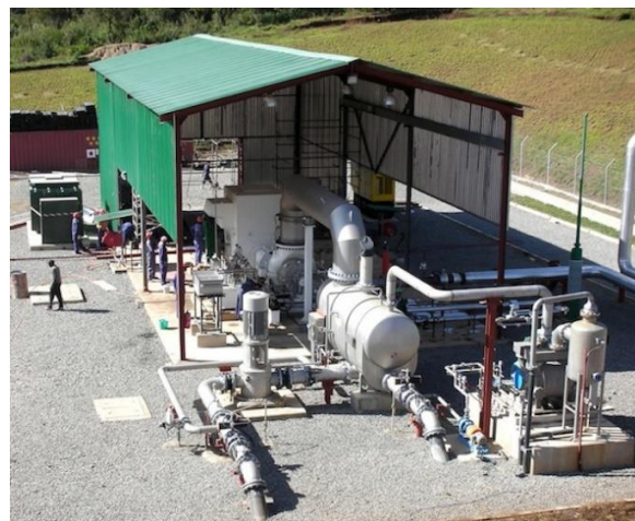
Figure 15: Photo of Eburru 2.4 MWe back pressure geothermal plant
