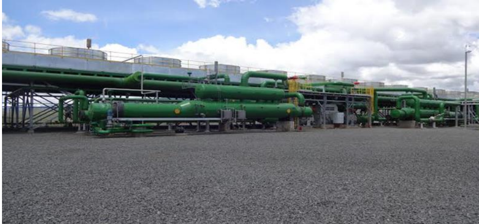
Figure 14: Orpower4 Power Plant at Olkaria III
