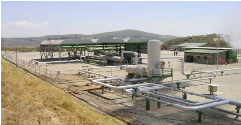
Figure 11: Photo of Oserian 2.5 MWe geothermal ORC power plant
