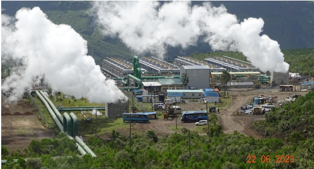
Figure 18: Photo of Sosian 35MWe power plant at Menengai. The plant uses Kaishan screw expander and ORC turbines
