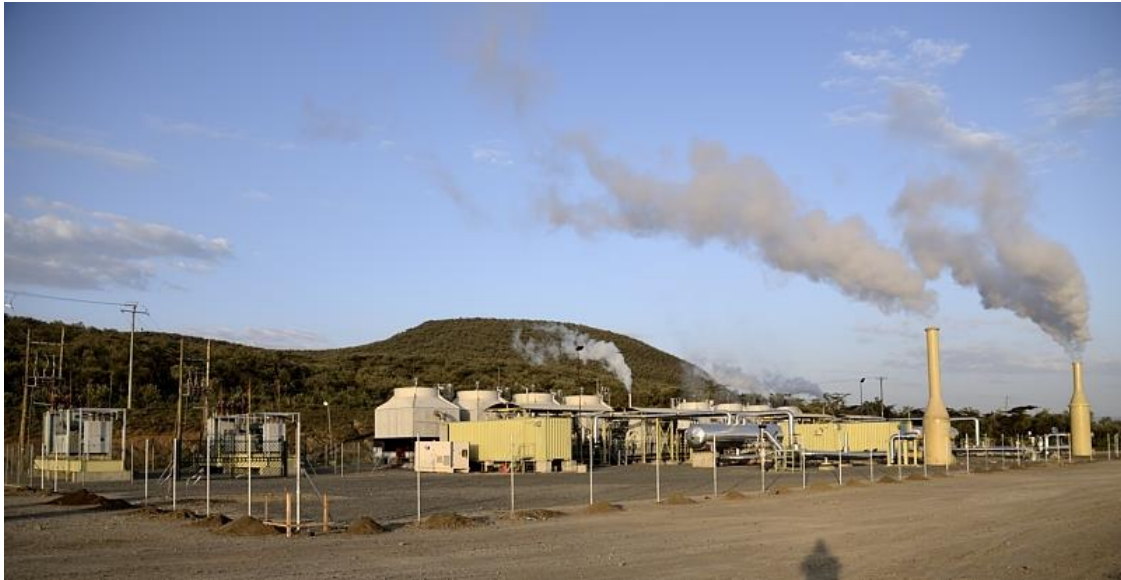
Figure 7: Wellhead power plants at Olkaria geothermal field
